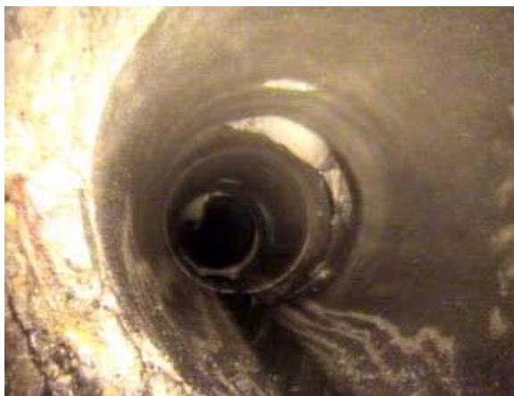
Figure 68 – (Photo 8) Joint décalé moyen
