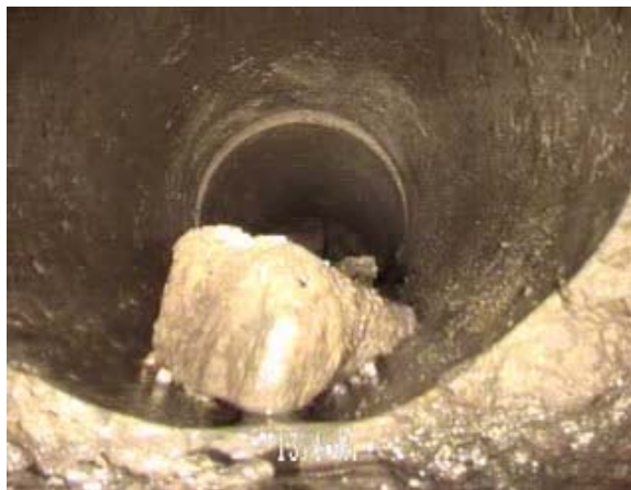
Figure 71 – (Photo 3) Raccordement obstrué
