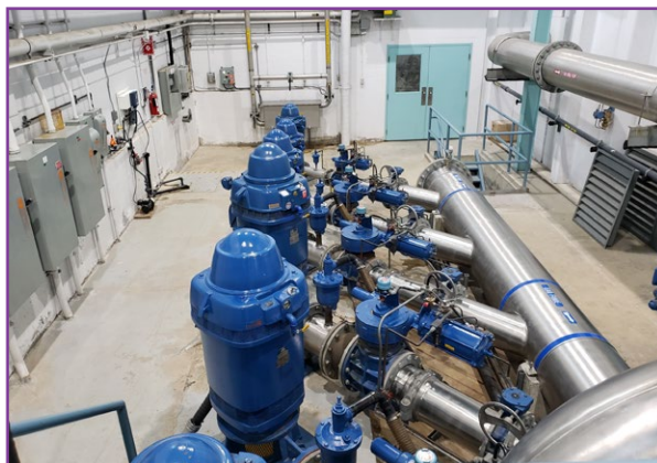
Figure 34 : Pompes de distribution (haute-pression)
